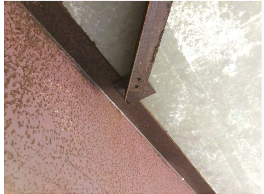
Bracing missing bolts
